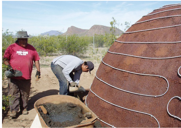
A DOMED STRUCTURE UNDER CONSTRUCTION MADE ALMOST ENTIRELY OF FERROCK. IMAGE © DAVID STONE
